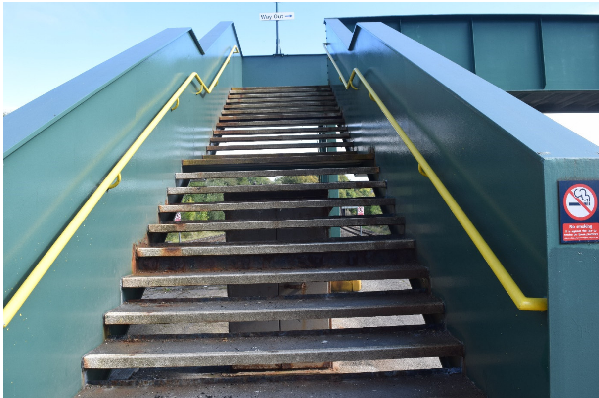
Photograph 7 –Open risers on Chinley Station footbridge
